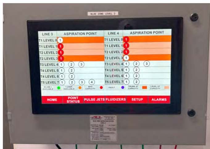
Vacuum drop control display indicating usage.
