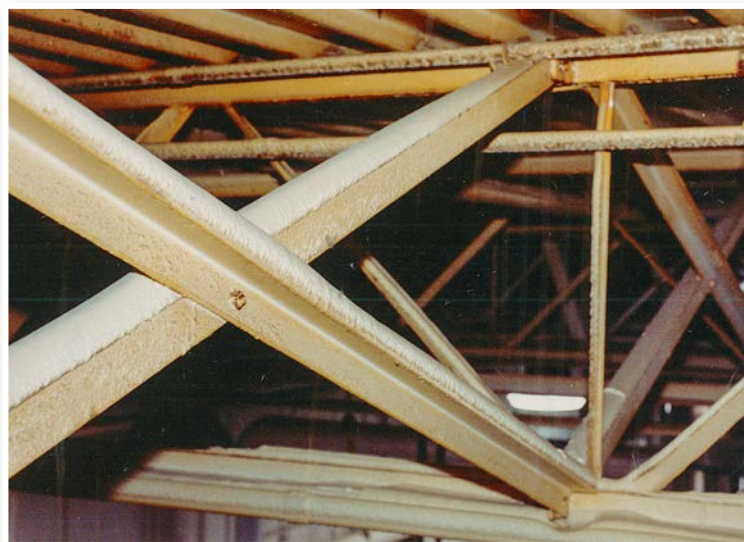
Corrosion danger from food salting after fryer cooking.
