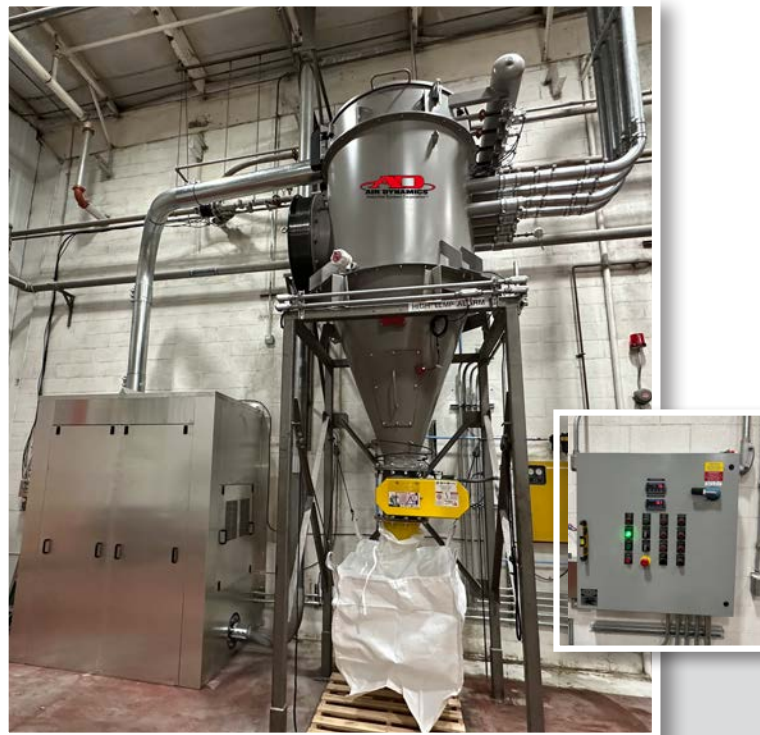
CV-48 Central Vacuum System with controls panel (inset).
