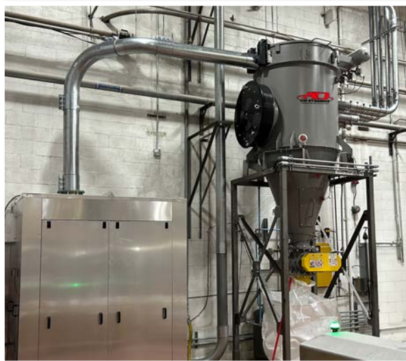
Air Dynamics CV-48 Installed.
