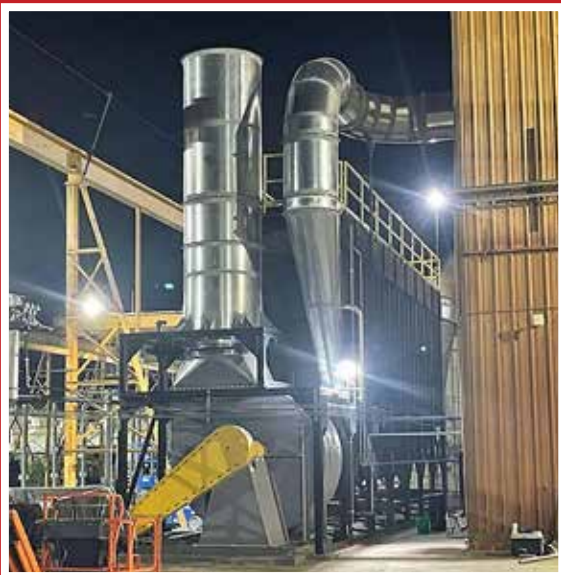
83,000 cfm dust collector.
