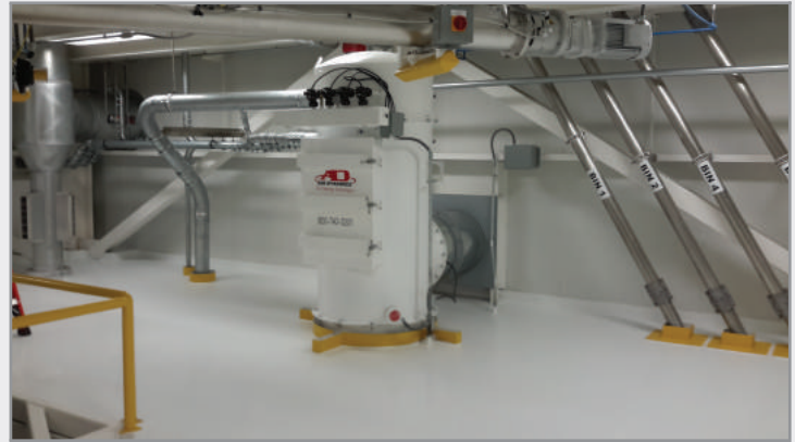
Central Vacuum System installed at MARS facility
